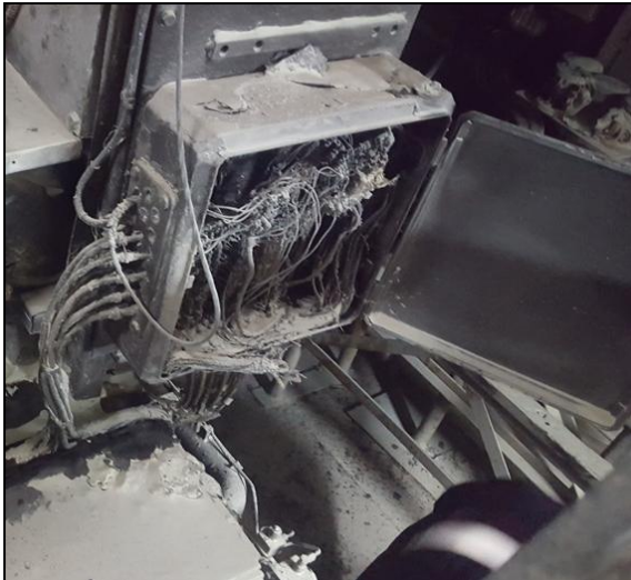
Figure 4: Damaged control cables
