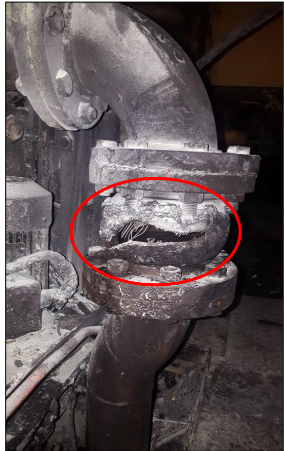
Figure 3: Damaged rubber bellows
